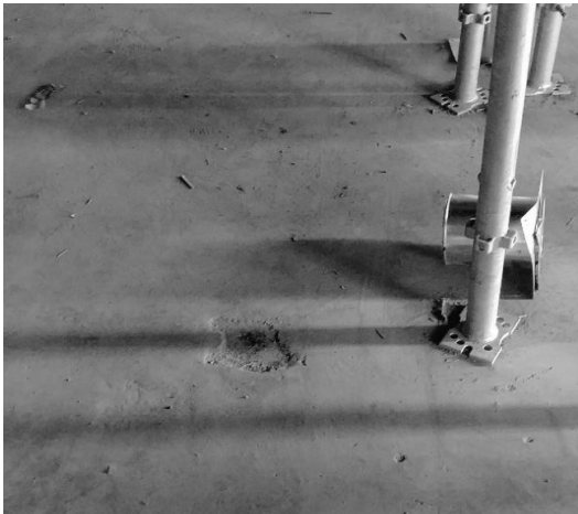
Figure 1: Floor concrete holes requiring patching work
