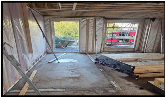
Figure 3: Rising wall too high
