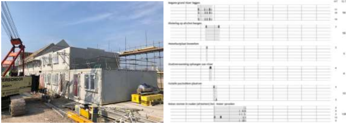
Figure 2a: Impression of site activities. 2b: Impression of the registration of activities.
