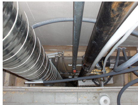
Figure 4: Left: DSM Illustrating Service Systems in A Generic Building. Right: Illustration of A Vertical Shaft with Different Media (Ventilation, Power Supply, Warm Water, etc.) Seen From Above.
