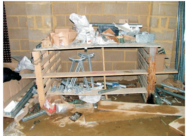
Figure 4: Improvised workbench and random storage of components.
