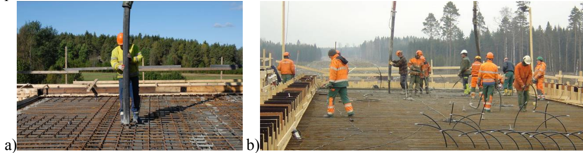
Figure 1: Typical Work Situation When a) Casting SCC. and b) Casting of Normal Concrete
