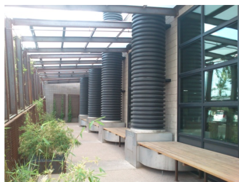
Figure 2: Evaporative cooling shower towers (Photo by Akash Ladhada, 10/22/13)
