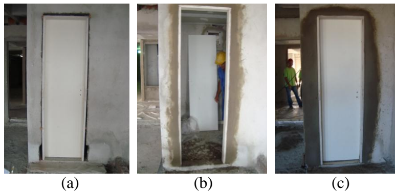
Figure 2: (a) Door frame permanently fixed; (b) Door is removed and frame remains fixed; (c) After the voids are filled with mortar the door is installed again.
