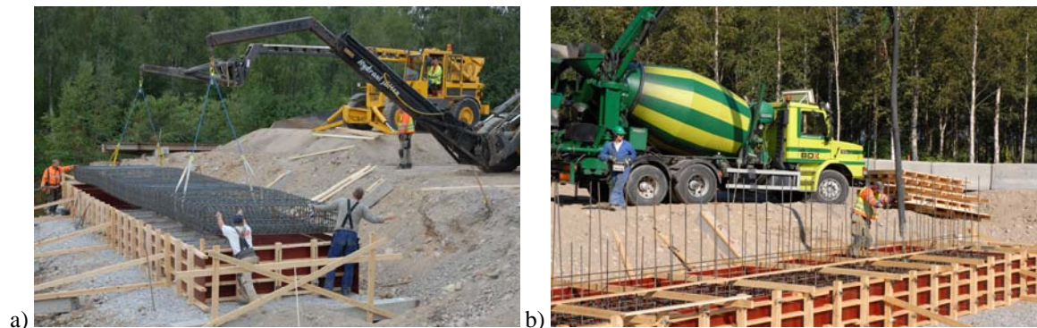
Figure 5 a and b: a) Placing the prefabricated reinforcement into the form work, and b) Casting of self compacting concrete for one of the foundations.
