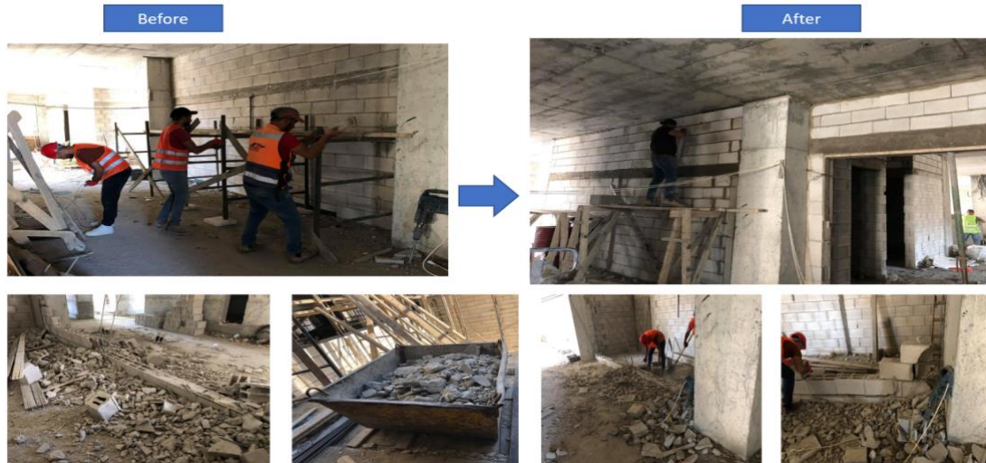
Figure 4: Lack of visualization for client review led to rework for a complete block wall
