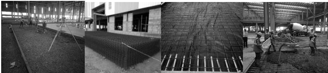
Figure 2: (a) Surface Levelling, (b) Reinforcement Mesh prepared in advanced, (c) LDPE Sheet and Reinforcement Mesh., (d) Concreting
