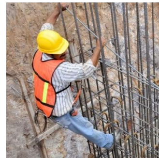
Figure 8: Working at a dangerous height with no Scaffolding
