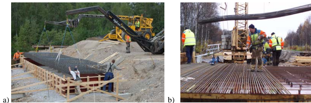
Figure 3: a) Placing prefabricated reinforcement for a foundation. b) Reinforcement carpet lifted into place.
