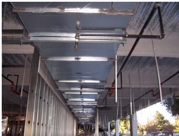
Figure 2: Example Priority Wall on Camino Project (photo courtesy of DPR Construction, Inc. Redwood City, CA)
