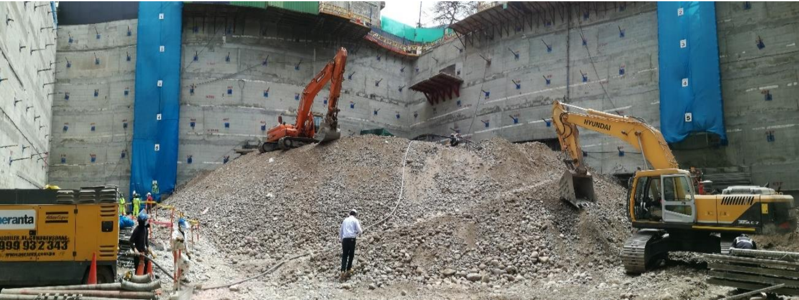
Figure. Set of material to remove that hinders the execution of anchored walls
